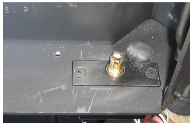
Illustr. 43: Door switch installed
