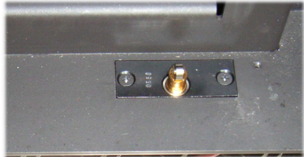
Illustr. 24: Door switch installed
